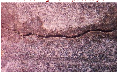
Moderate cracking, up to ¼" wide, slight faulting or impact on flow
