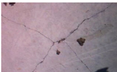
Mild cracking, no impact to flow
