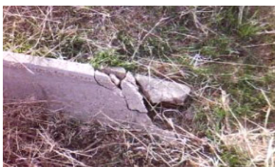
Mild damage to outlet
