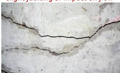
Severe cracking, wider than ¼", with significant faulting
